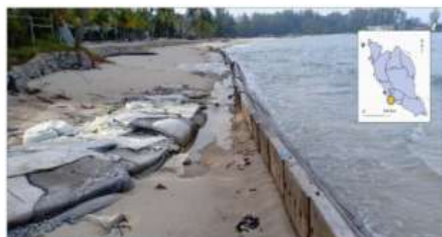
Fig .4 . Sediment loss in coastal areas
